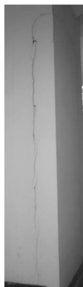
Figure 31: Vertical crack in a pillar (South West apse, Saint-Vincent Church)
