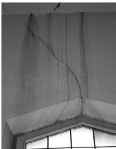
Figure 30: Crack in the central part of the beam above the by lighting the gallery (East front, Saint- Vincent Church)
