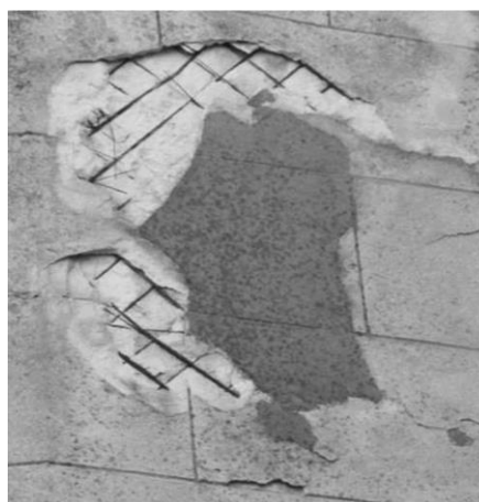
Figure 36: Typical spalling inside Pauchot reinforced artificial stone, North West apse, Saint-Vincent Church
