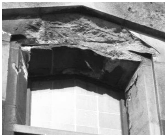
Figure 34: Spallings around a North bay, Saint-Vincent Church
