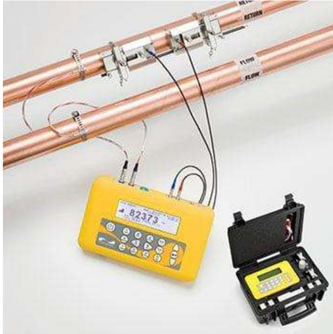
Fig. xxx: Ultrasonic flowmeter measurement (source: Micronics documentation)
