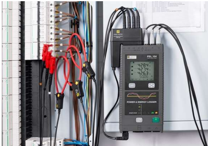
Fig. xxx: Wattmeter measurement (source: Chauvin Arnoux documentation)
