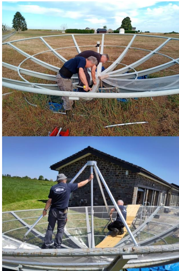
Figure 4: Top: Early measurements on the parabola for new rings; bottom: the new rings, mesh and feed support being installed
