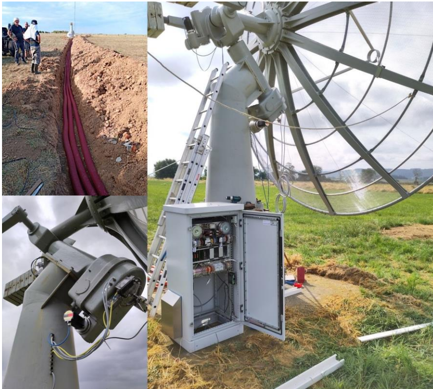
Figure 6: Top right: trenches carrying pipes for the power supply, one optic fibre for the network, and 2 optic fibres for RF over fibre; bottom left: motors and cabling on the mount; right: view of the control rack with its electronics and computer
